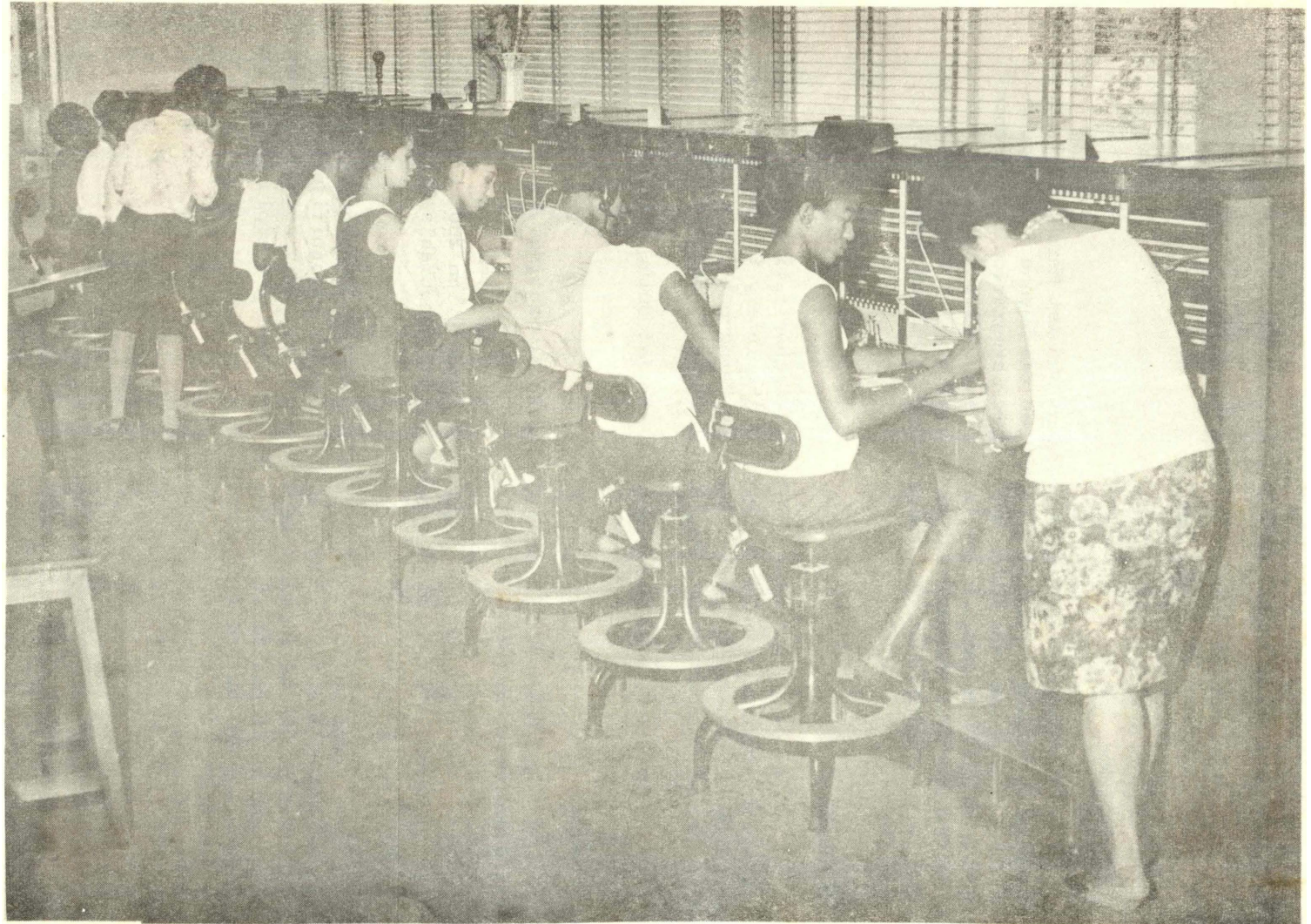
A Section of the Operating Staff on the Manual Switchboard in the Georgetown Exchange.
