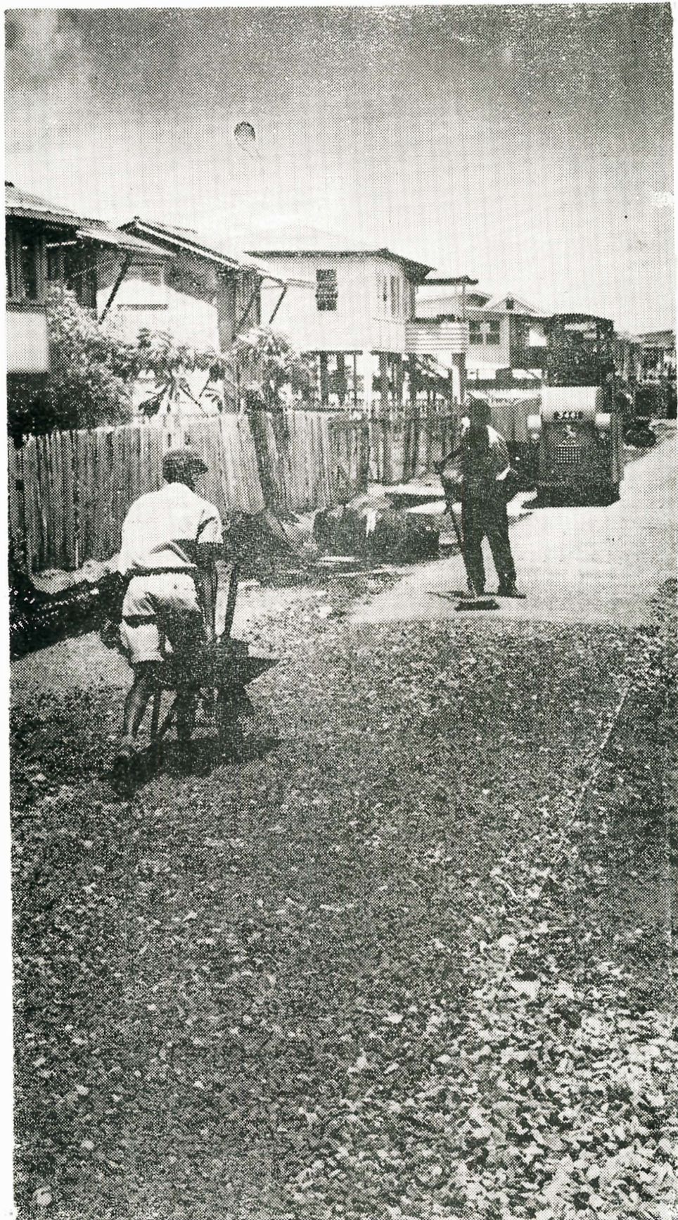
Asphalt-bound gravel road under construction in the Annandale Extra Nuclear Housing Area, Lusignan Estate.
