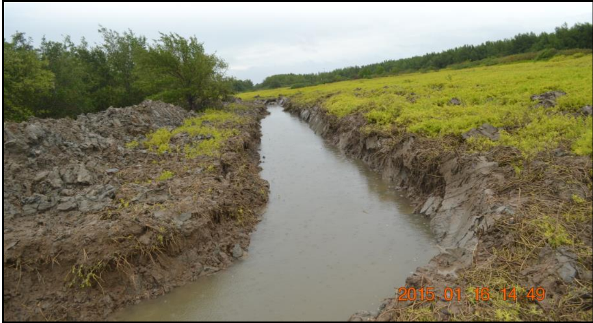
Figure : Channel at Wellington Park completed as part of the Hydrologic Restoration
