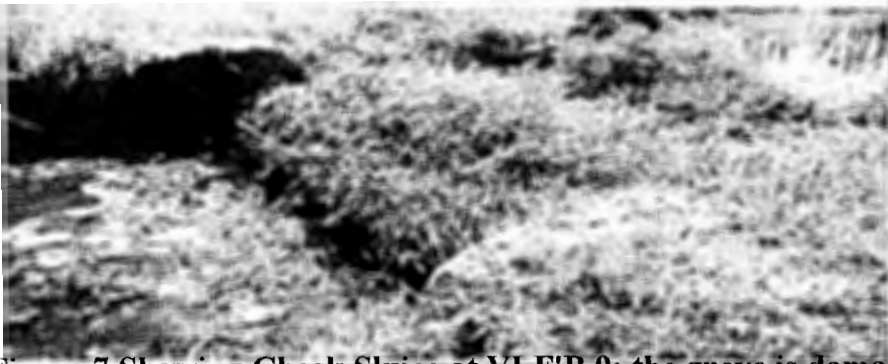
Figure 7 Showing Check Sluice at VLF'B 9; the grove is damaged and can't hold the planks securely; hence, this had to be supplemented with a Mud Stop-off to keep the water out of the block
